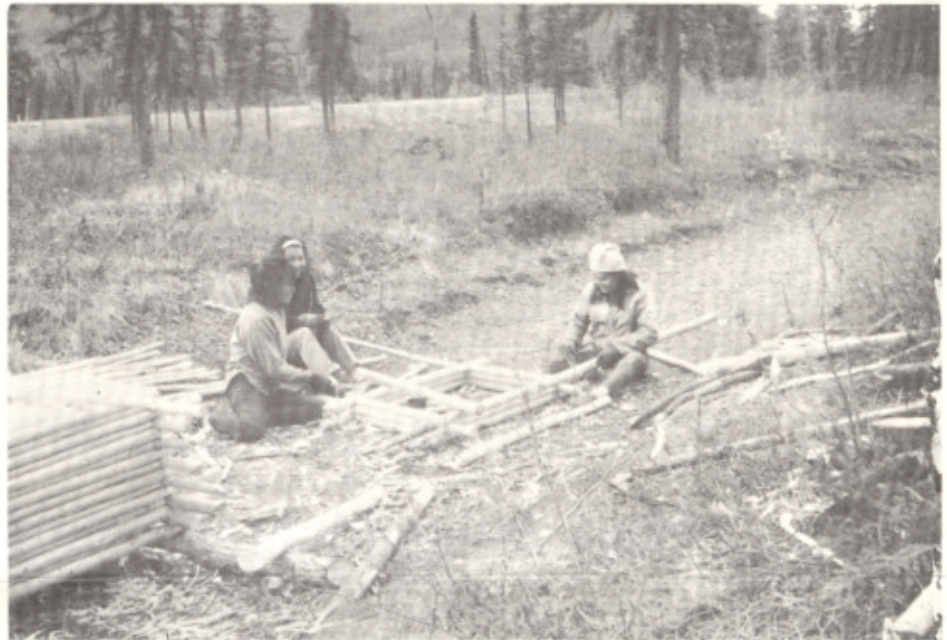
Building a cache and dog houses calls for peeled logs and yards of peeled spruce roots. These women workers are refining their knowledge of traditional Indian crafts in constructing an authentic Indian village near Mentasta.
