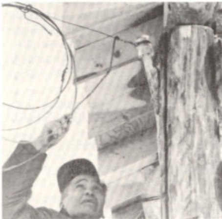
Attaching wiring to an insulator is part of the Copper Center telephone system.
