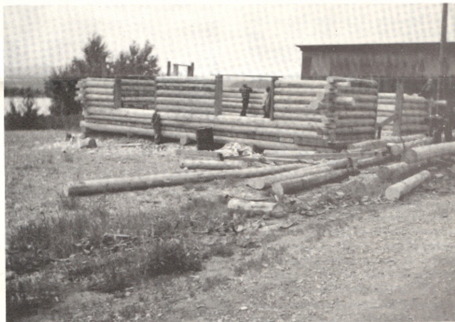
Massive logs will form the new Klukwan Tribal House, due for completion later this year. Operation Mainstream is paying wages of a construction crew from the village, with materials donated by villagers, and the Haines Lumber Company.
