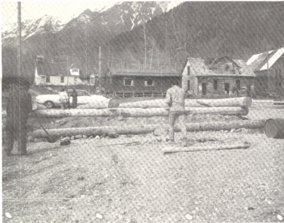
Foundation work begins in Klukwan to re-build a Tribal Community House where villagers can display their arts and crafts. In the photo above workers are laying logs for the new foundation.
