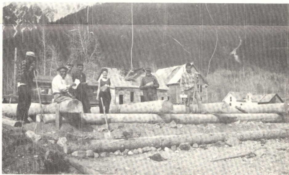
Dedicated workers have put in foundation logs for their new Tribal Community House. Mrs. Dorothy Fossman, Tribal House superintendent looks over the progress, and admires the work.
