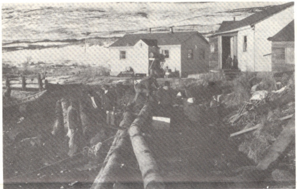
This picture shows the poor condition of the bulkhead, with the center section completely missing and all the fill gone behind the section in the foreground. The boat at the far left is left setting on dry ground during low tides.
