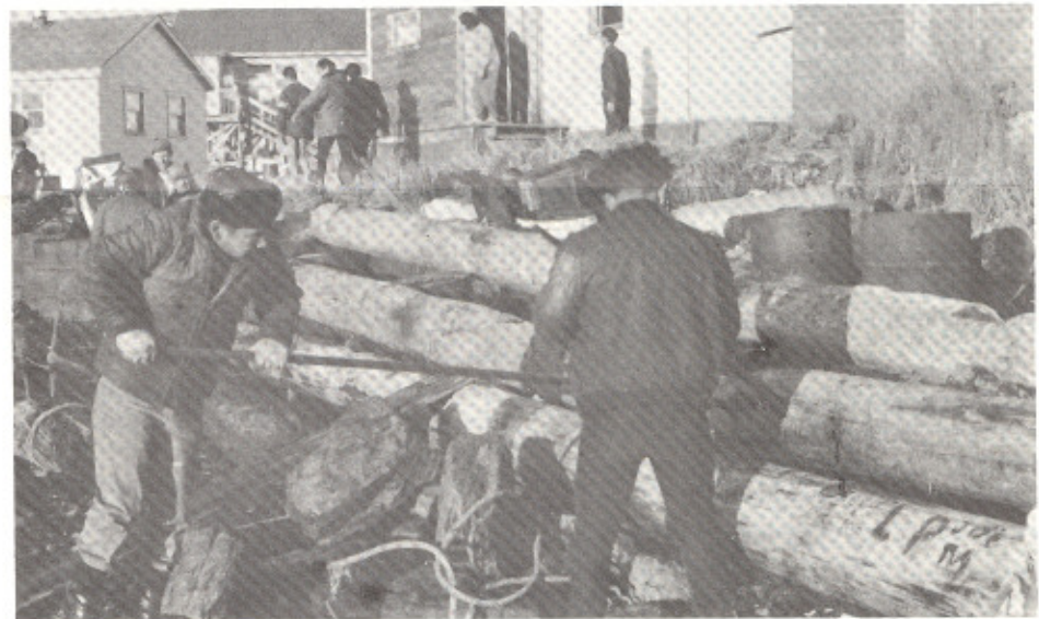
Two men work on reconstructing the damaged bulkhead at Akhiok. Directly behind the bulkhead are several homes which have been victims of high tides in the past. The new bulkhead will be higher and more sturdy than the last
